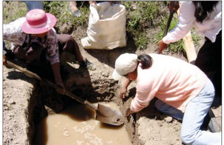
Above: Villagers dig a well in Raric that allows the testing of water quality with a perc test, which will help the EWB-UMD team evaluate the potential potable water resources in the area. The water was tested for Ph, iron, alkalinity, hardness, chlorine, nitrite and nitrate levels.
