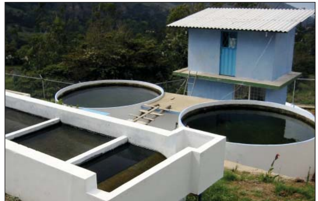
Above: A functioning water sanitation facility in a village near Uduzhapa and Raric, built by a previous EWB-UMD group led by Dr. Peter Chang of Civil Engineering. The team hopes to build smaller facilities in Uduzhapa and Raric, Guatemala.
